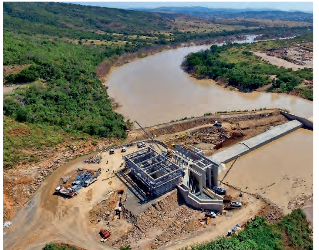
The Lower Thukela Bulk Water Supply Scheme is expected to be fully functional by the first week of November.
